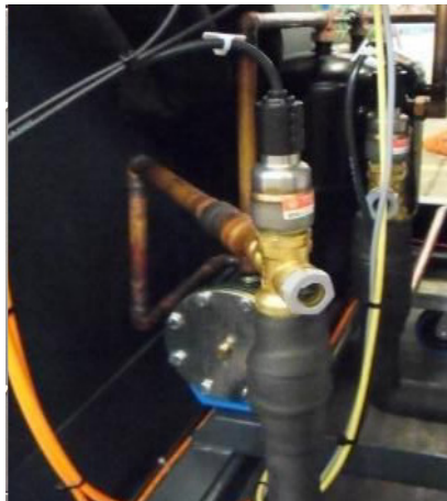
Valvole termostatiche elettroniche Electronic Expansion thermostatic valve.
